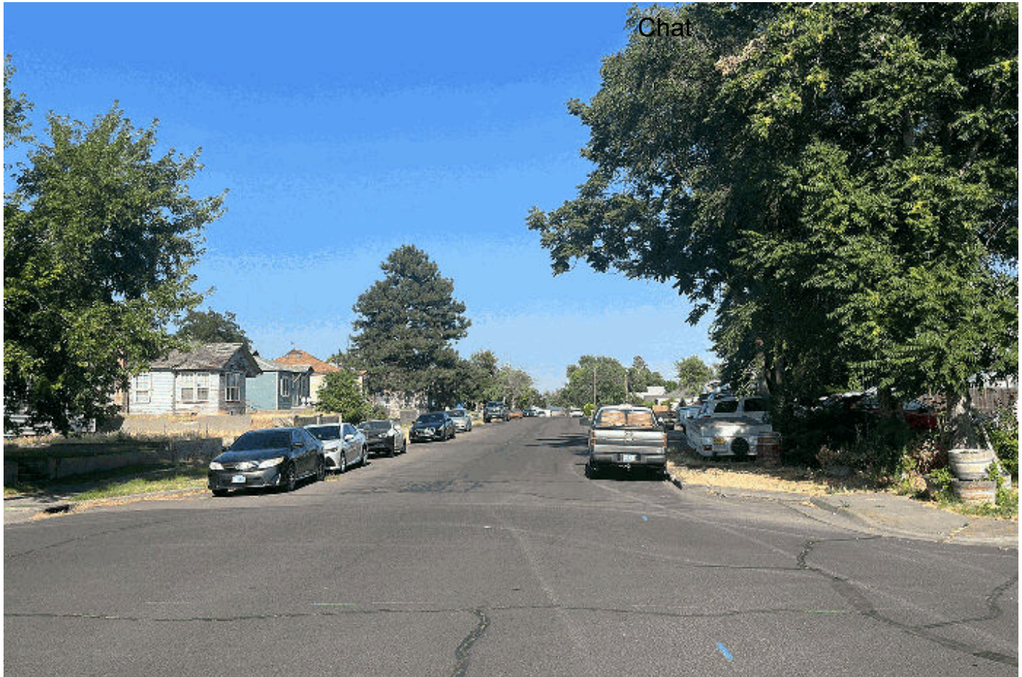
Crews are replacing aging water mains along several streets in Hermiston beginning July 16, 2024.
